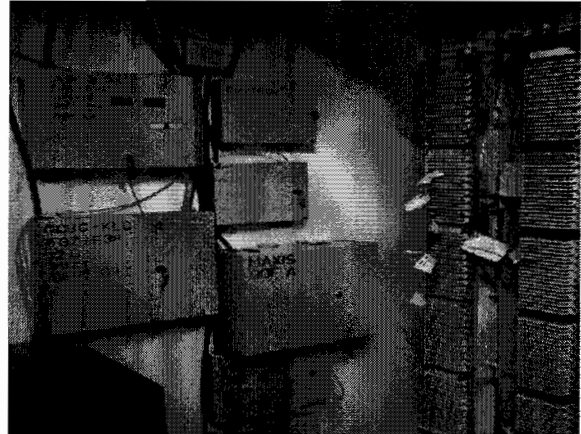
MDF room of a building where we performed inside plant installation and commissioning services
